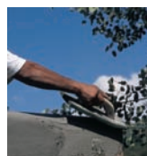
1. Coating the surface with a repair and base-coat product such as Sto Flexyl to fill cracks and waterproof
