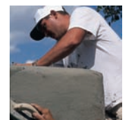
4. Smoothing out the surface so the repair is not visible after the finish coat is applied
