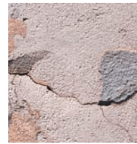
Damage due to cracking or moisture getting below the surface
